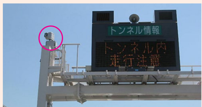
Pan-tilt camera for monitoring the tunnel entrance/exit (in the circle)
