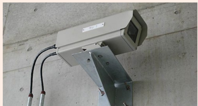
Fixated camera for preventing disaster in the tunnel
