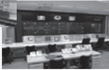
Train Radio Communication Systems
