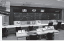
Train Radio Communication Systems
