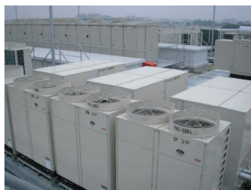
An Ice Thermal Storage Air Conditioning System was installed in the new building at Koganei Works. This earth-friendly air conditioning system reduces CO 2 emissions that cause global warming thanks to the use of night electricity with less fossil fuel.
