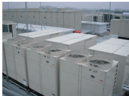
An Ice Thermal Storage Air Conditioning System was installed in the new building at Koganei Works. This earth-friendly air conditioning system reduces CO 2 emissions that cause global warming thanks to the use of night electricity with less fossil fuel.
