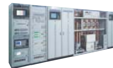
● Water-cooled 3kW Digital Terrestrial Broadcasting Transmitter Transmitting systems at key stations, which transmit terrestrial digital TV broadcasting waves
