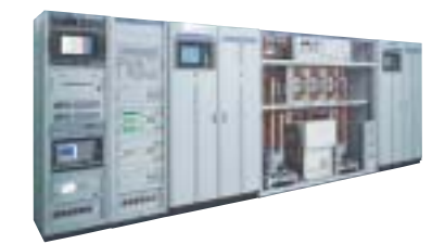
● Water-cooled 3kW Digital Terrestrial Broadcasting Transmitter Transmitting systems at key stations, which transmit terrestrial digital TV broadcasting waves
